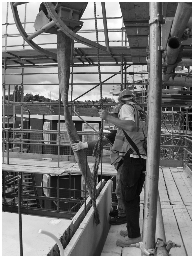
Figure 8. Placement of SCC into a confined space removes the difficult task of compacting (courtesy of Lafarge)
