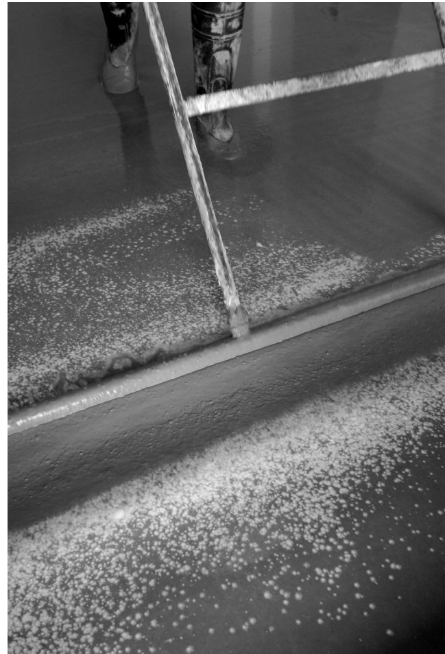
Figure 7. Simplified placing, dapping to a finish, reduces the impact on operatives (courtesy of Lafarge)
