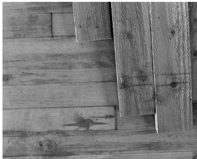
Figure 9. Reflection of timber formwork material on final finished face of an SCC wall (courtesy of Lafarge)
