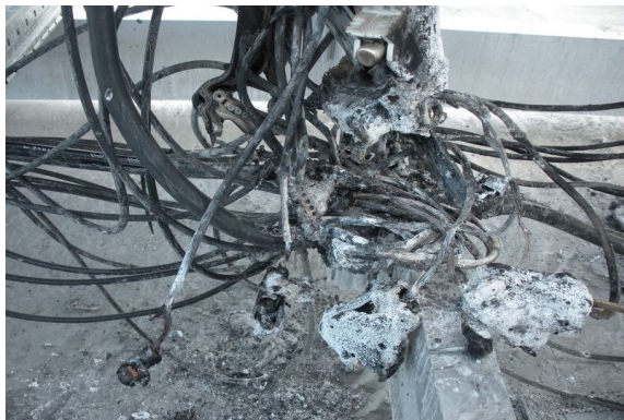
Figure 1: Charred remains of a DC junction box where a fault combined with incorrect fuse installation has caused a fire.
