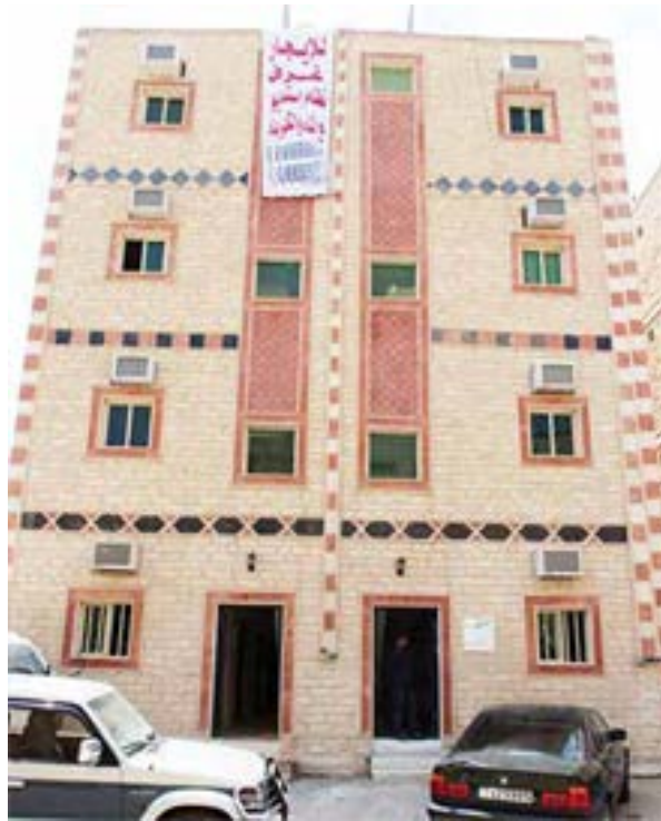
Fig. 3.55: A House (in Julib ALShuokh) has four floors in violation with BR 1985
