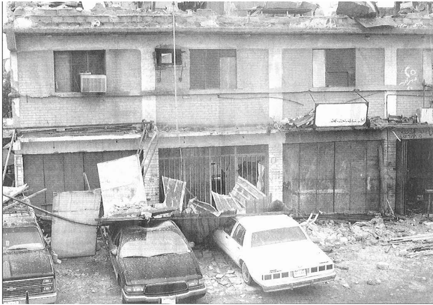
Fig. 3.47: Part of Building Collapse on January 2004 at Kuwait
