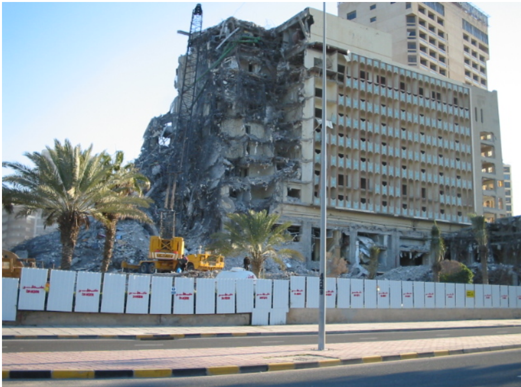
Fig. 3.32: Destruction of Hotel Safir, Kuwait City (photo by the author - 2004)
