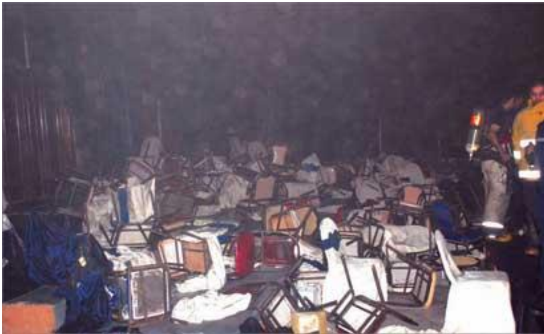
Fig. 3.41: Fire of merrymaking building in April 2009
