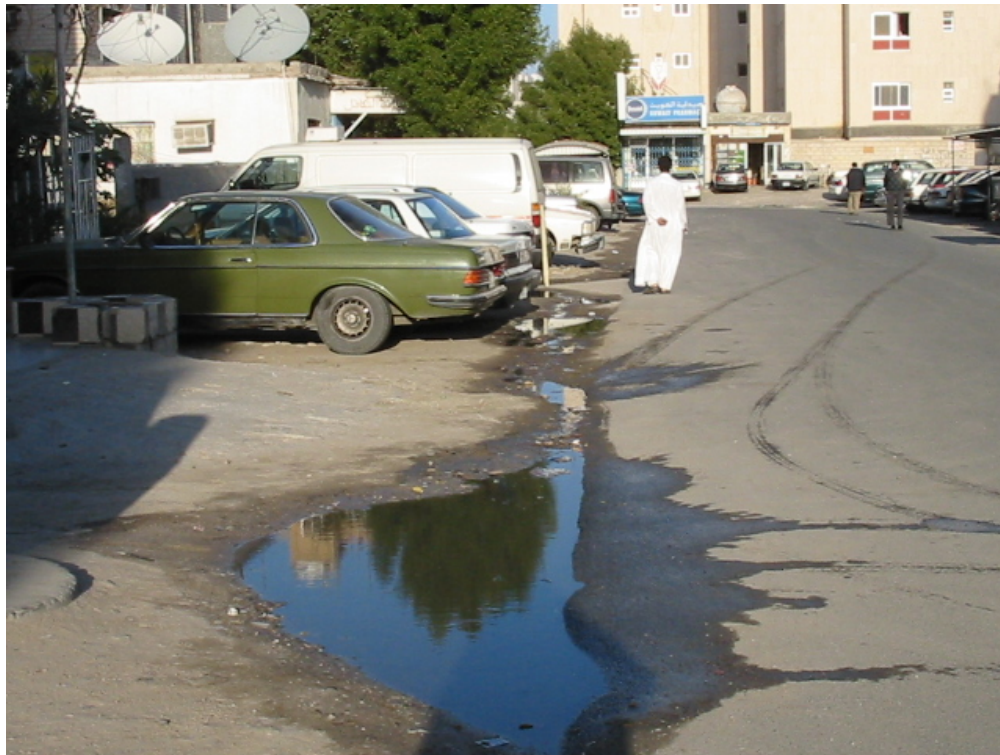
Fig. 3.29: Problems of grading and drainage of exterior property areas
