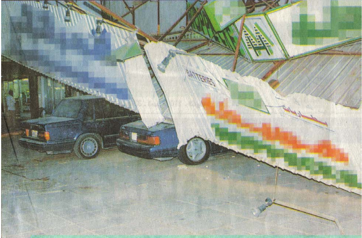
Fig. 3.22: Fall of cars' metal shed
