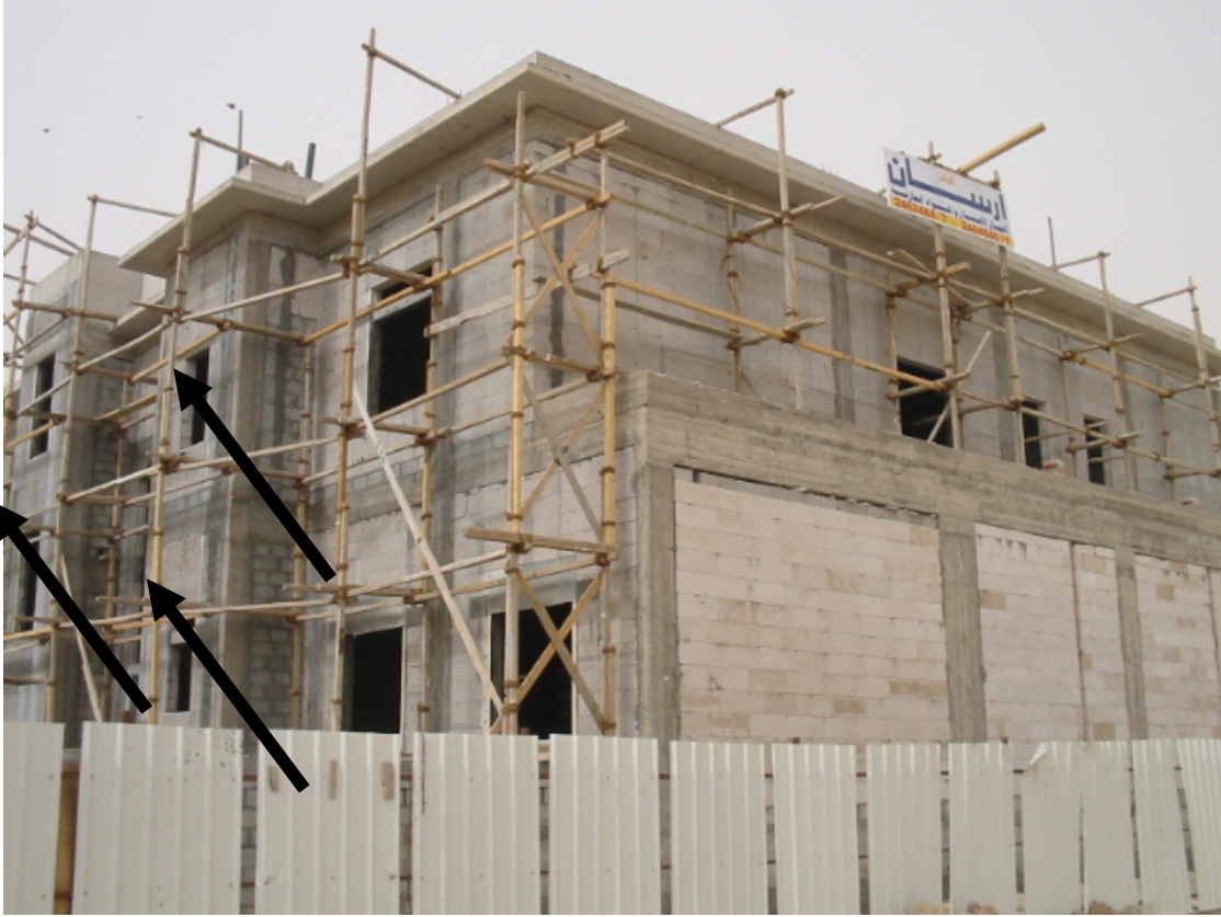
Fig. 3.57: Side View of Villa showing violate code by filling up parts of walls with non insulating bricks
