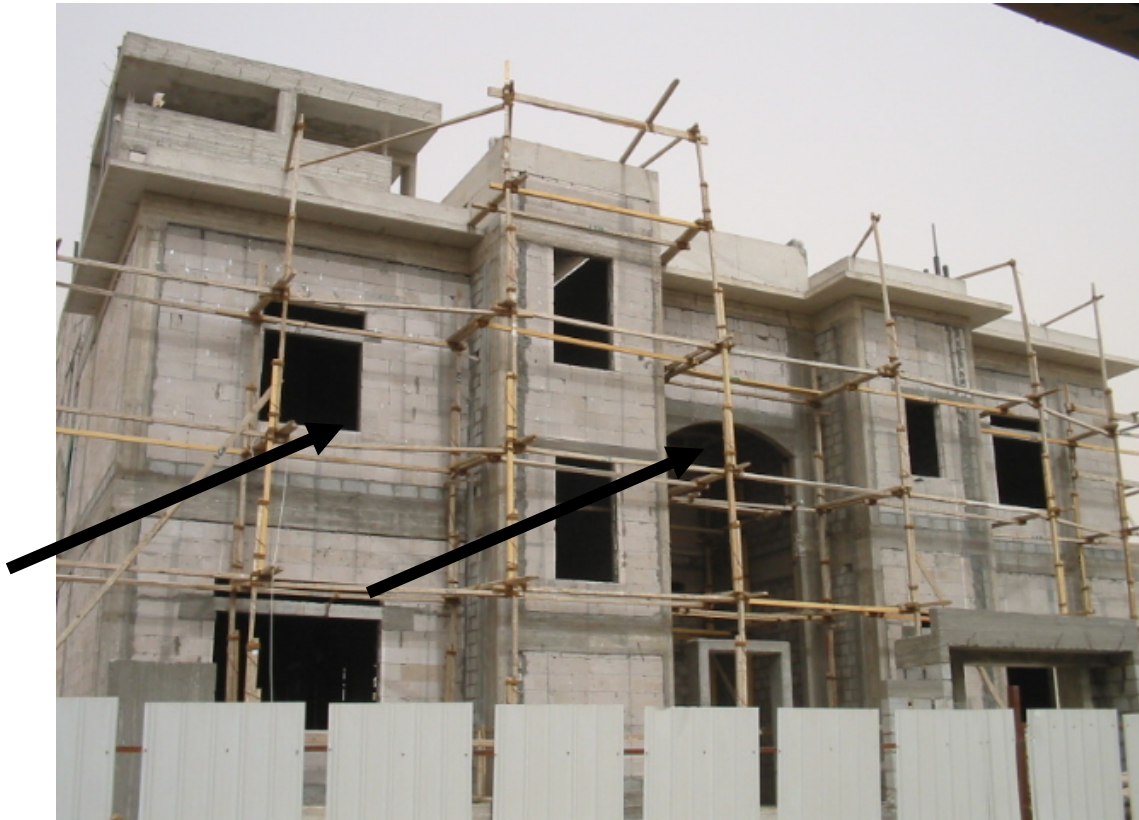
Fig. 3.58: Front View of Villa showing violate code by filling up parts of walls with non insulating bricks
