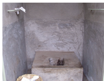
Figure 5. Raised toilet seat with handrails on side walls 6
