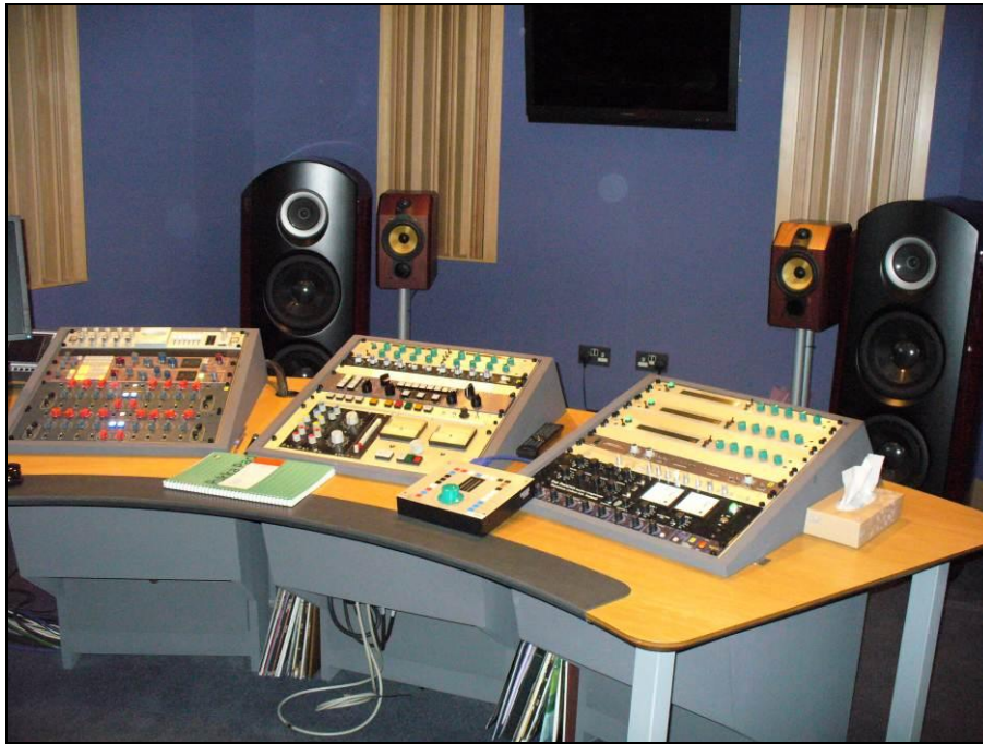
Figure 5-7: Mastering studio showing consoles and monitoring speakers, Air Studios, North West London
