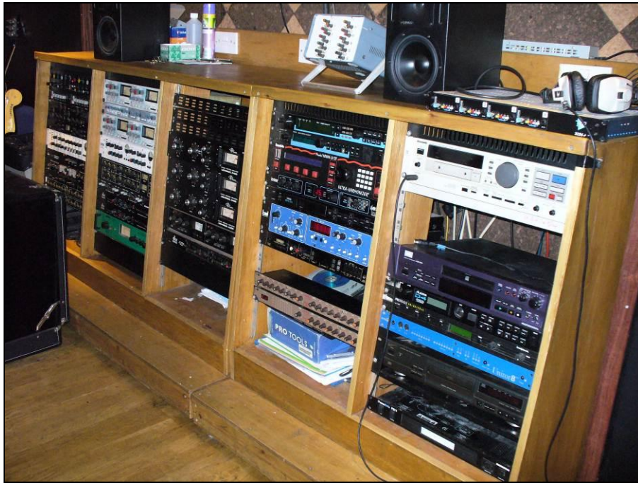
Figure 5-13: Rack of outboard equipment including preamplifiers and effects units, Fortress Studios, North London
