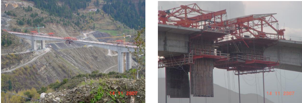
Figure 3: Views of under construction Metsovo ravine bridge, (a) General view, (b) key of central span.
