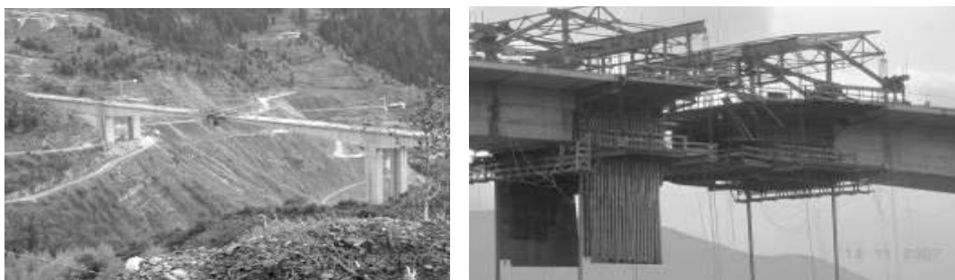
Figure 2. Views of under construction Metsovo ravine bridge a) General view b) key of central span.
