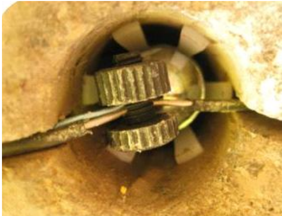
Figure 4 A galvanic anode with a titanium connection temporarily fitted in a hole.
