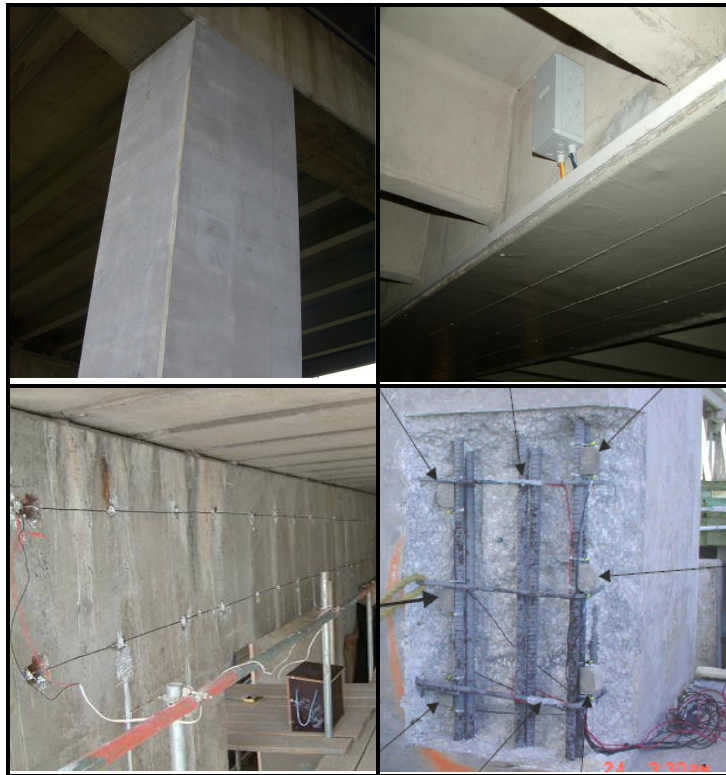
Figure 4: Sacrificial anode examples including a thermally applied metal coating (top left), adhesive zinc sheets (top right), discrete anodes in drilled holes (bottom left), discrete anodes installed in patch repair (bottom right) (Dugarte et al. 2007).
