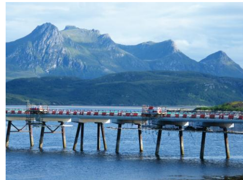
Figure 10 Tongue bridge during the installation of a hybrid electrochemical treatment on the concrete substructure.
