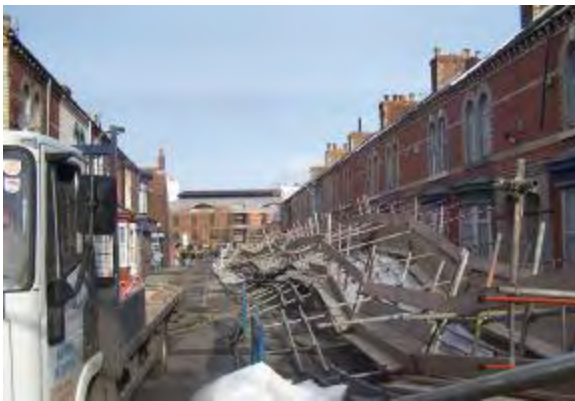
Teeside scaffolding collapse, 2008 (courtesy HSE)
