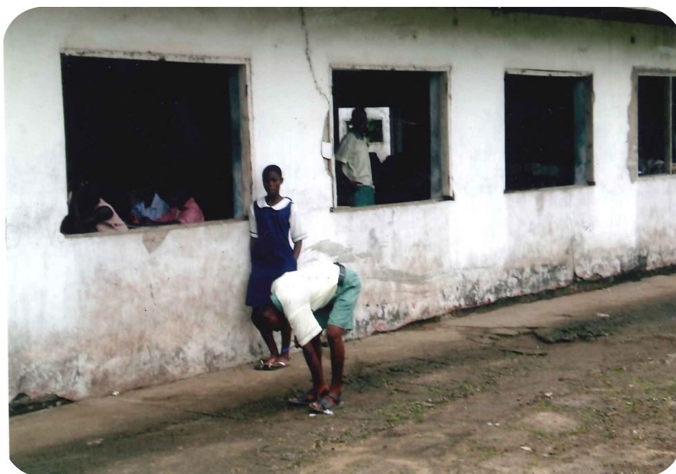
Picture 7.6: The Deplorable State of Classrooms Built Without Windows
