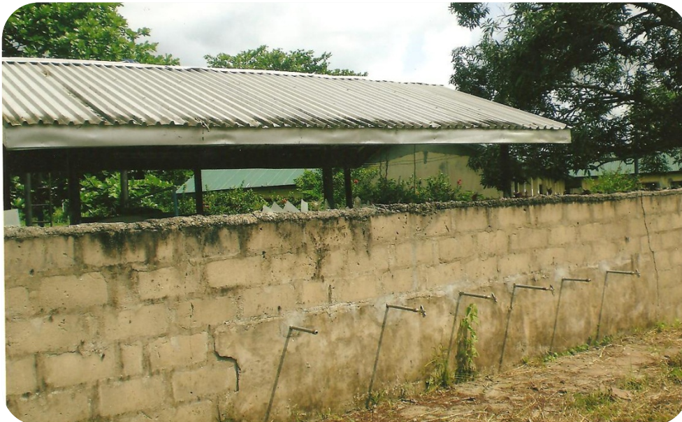
Picture 6.3: Non-functional Water Pumps in Ogbolomai Community, Bayelsa State
