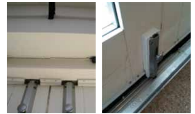
Figure 2a & 2b: Door and window perimeter seals: (a) as installed by contractor with gaps & (b) reinstalled with continuous seal
