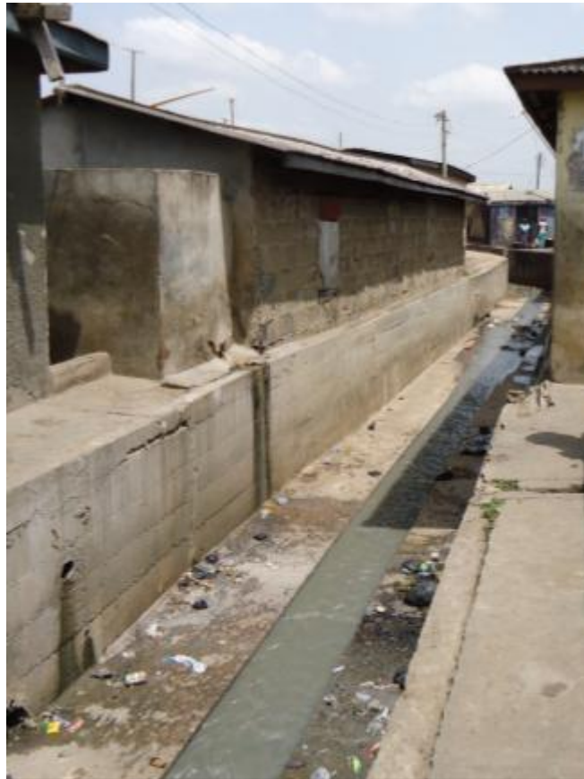
Figure 10-11 Main drainage channel in Nii
