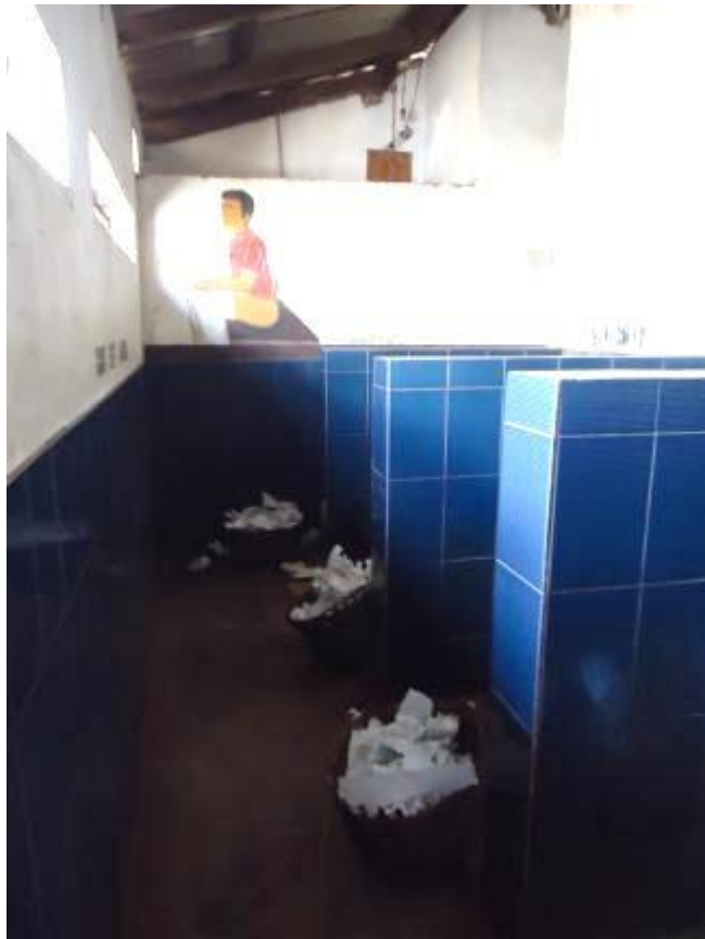
Figure 10-27 Men' cubicles in a commercial shared toilet in Oko
