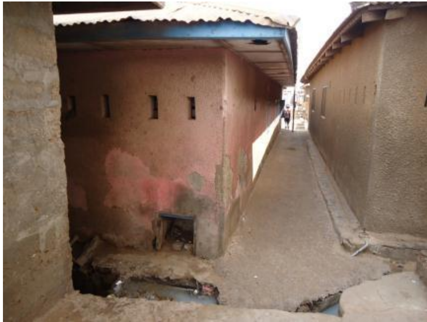
Figure 10-18 Closed down bucket toilet of a compound house in Nii
