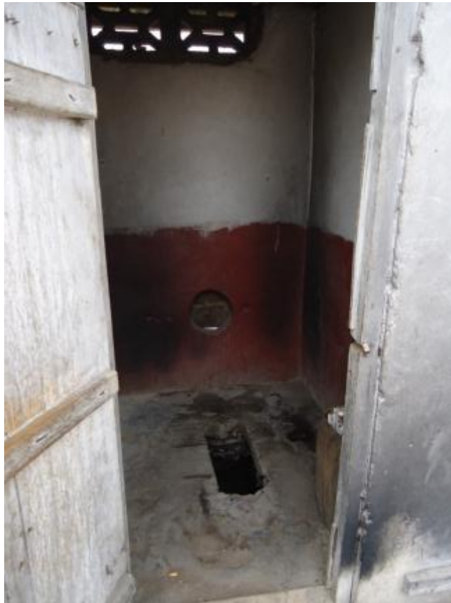
Figure 10-28 Cubicle in a neighbour shared toilet in Amui
