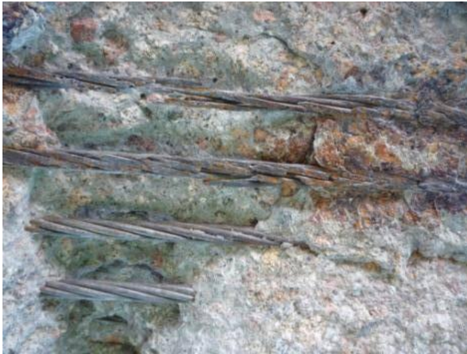
Figure 3: Typical chloride induced deterioration of the prestressed concrete beams
