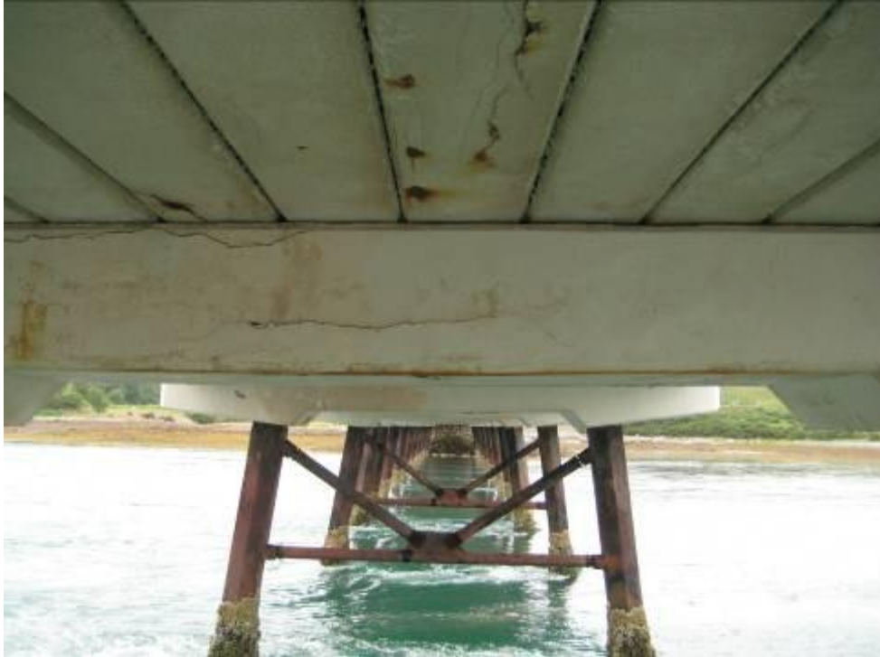
Figure 4: Typical chloride induced deterioration of the bridge
