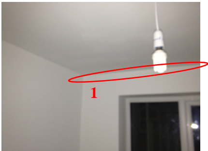
Figure 64. Photograph of the interior of plot 7 northerly bedroom ceiling line at the cedar cladding height.
