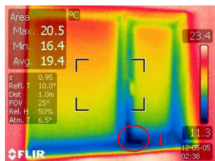
Figure 67. Internal infrared image west facing bottom flat window dwelling 7
