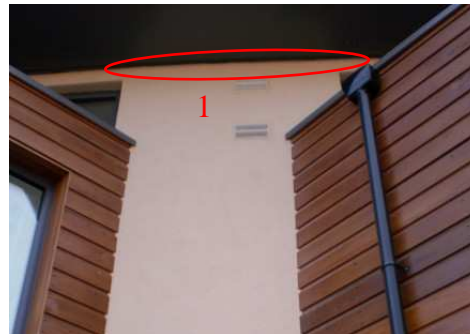
Figure 72. Photographic image of the exhaust of heat recovery unit from the houses.
