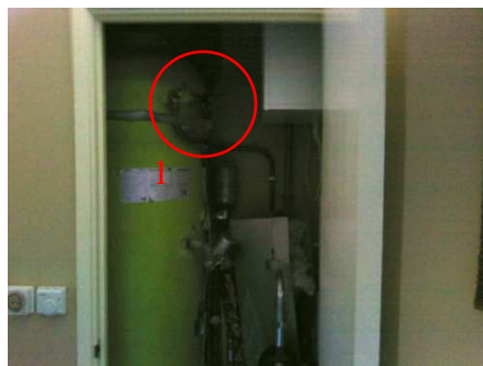
Figure 76. Photograph of the thermal store.
