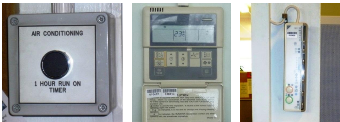
Figure 4.8 Examples of easy to understand and less intuitive temperature controls in the County Council buildings
