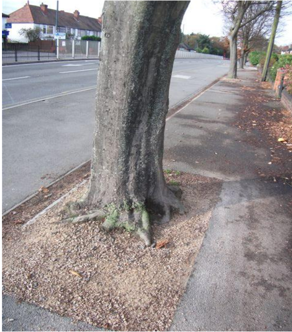
Fig 103; Example of poor pavement condition
