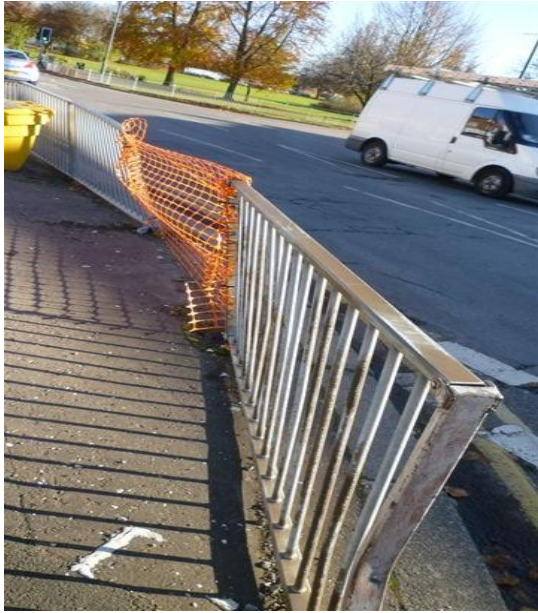
Fig 110; Guard rail damage, Daventry Road
