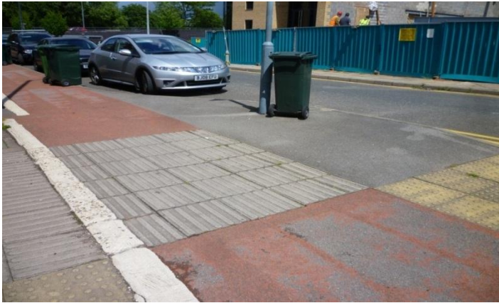
Fig 65; Example of damaged paving
