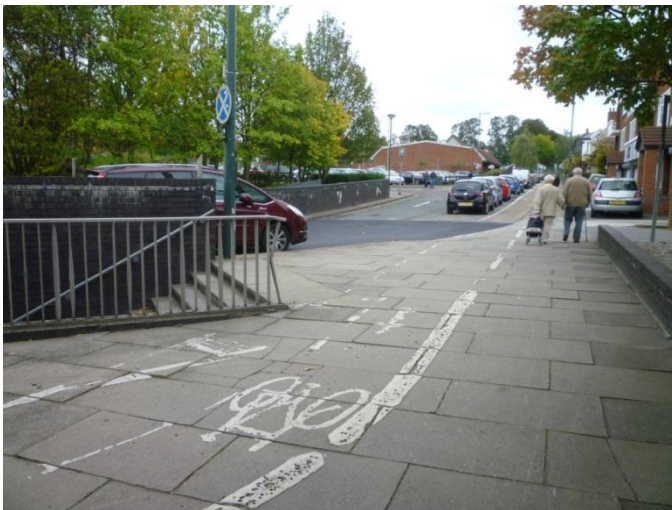
Fig 69; Inadequate marking of pedestrian/cycle paths, with degraded pavement markings
