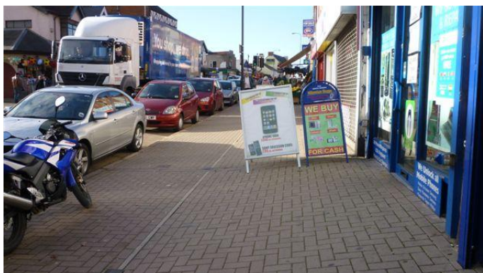
Fig 122; Pavement condition, Walsgrave Rd (2)
