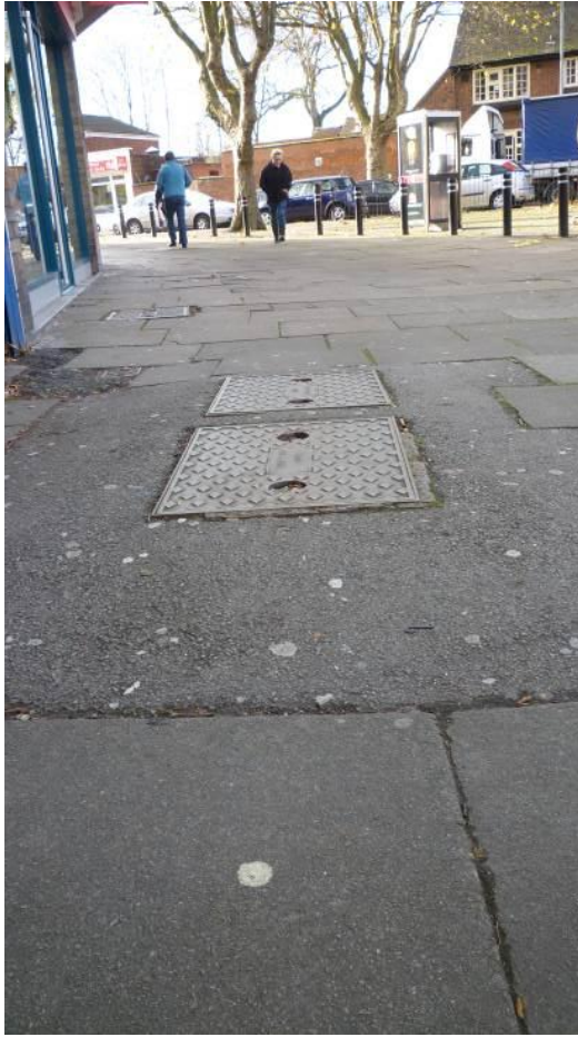
Fig 120; Poor pavement condition, Walsgrave Rd (3)
