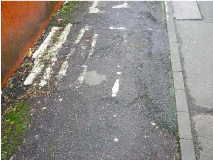
Fig 68; Unclear marking of pedestrian/cycle paths, with degraded pavement markings
