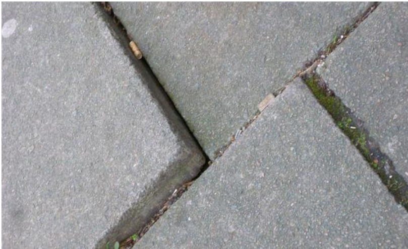
Fig 118 Poor pavement condition, Walsgrave Rd (1)
