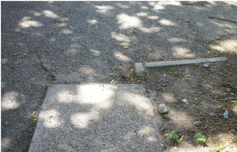
Fig 64; Example of damaged paving
