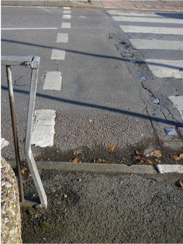
Fig 109; Poor pavement condition at Quinton Rd crossing
