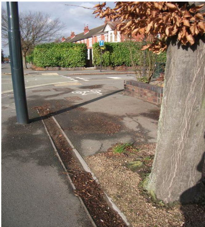
Fig 104; Example of poor pavement condition
