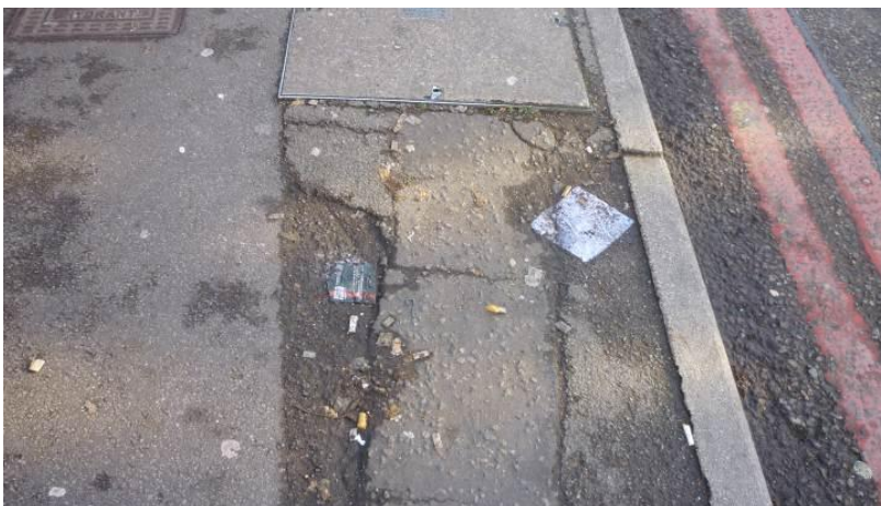
Fig 119; Poor pavement condition, Walsgrave Rd (2)
