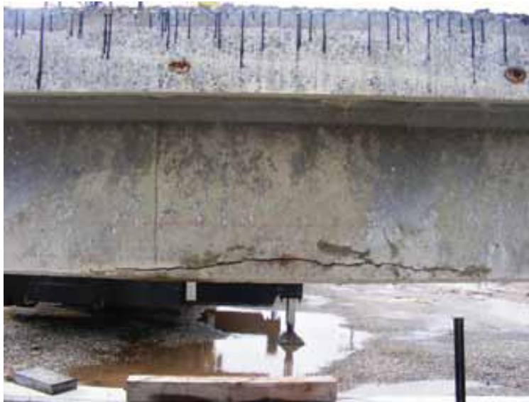
Figure 5 Typical chloride induced deterioration of the superstructure.
