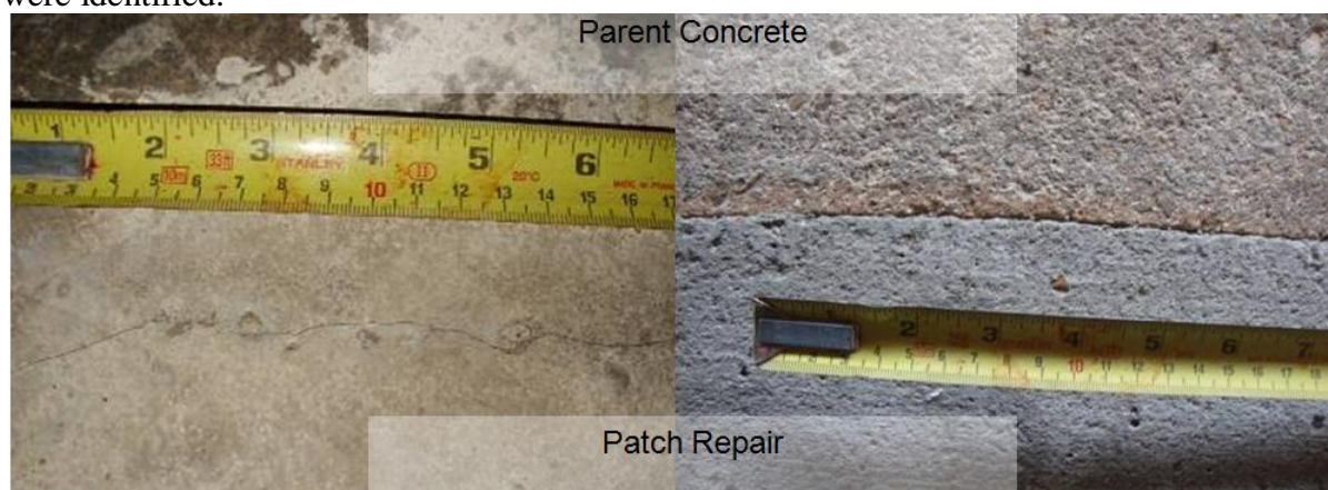
Figure 7: Cracks at the interface of a patch repair in the car park using material A, before and after surface preparation with mechanical shot-blasting
