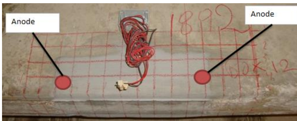
Figure 7: Typical galvanic anode installation at monitoring station to facilitate galvanic current measurements.
