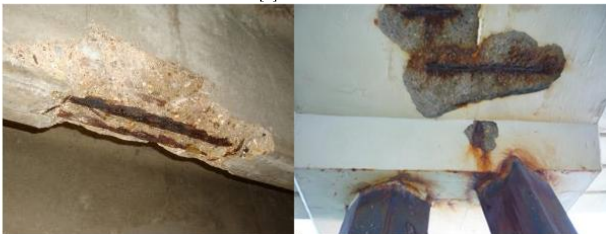
Figure 5: Chloride-induced corrosion and spalling to the MSCP and bridge structures (respectively)
