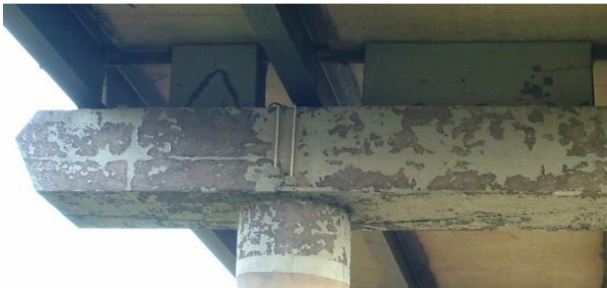
Figure 3: Beam tested for long term effects of ICCP, showing evidence of severe anode deterioration but not signs of corrosion
