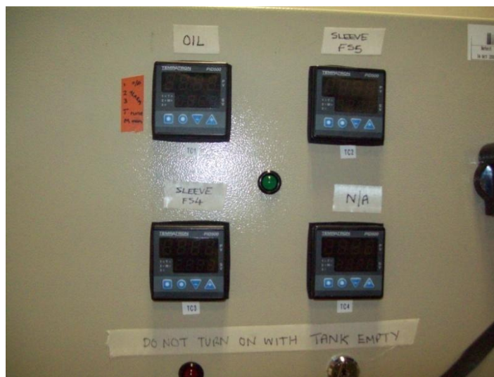
Figure 4-7: Temperature Setting on the Heater System Control Panel
