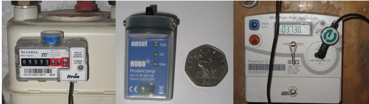
Figure 3: From left to right – gas meter fitted with pulse module, hobo pendant sensor used for temperature monitoring and electricity meter fitted with LED pulse detector.
