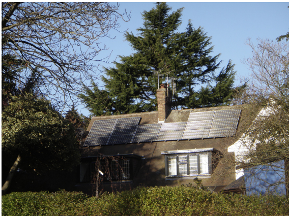
Fig. 1. Photograph showing a south facing PV-system which is not heavily shaded but the energy yield loss due cell mismatch is significant.
