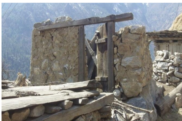
Figure 6-29 One of many latrines in disrepair in Chaggaunphaya (Author, 2012)
