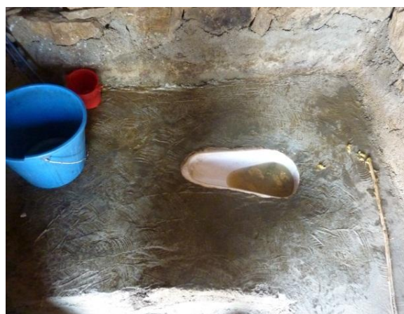
Figure 6-10 A blocked latrine from use of stones for anal cleansing (Author, 2012)
