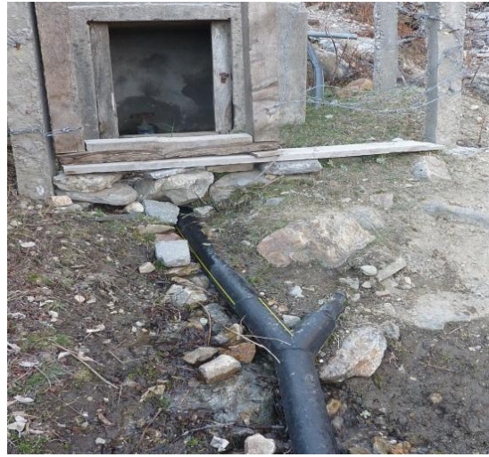
Figure 6-3 Exposed pipe was found to be commonplace both at the source and between the source and the outlet (Author, 2012)
