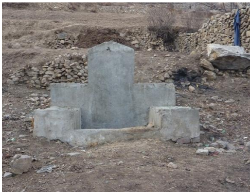
Figure 6-34 One of the broken taps in Ward 1 – these taps delivered water for one day only (Author, 2012)
