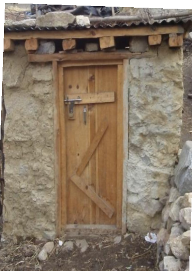
Figure 6-8 A modern government provided offset pour flush pit latrine (Author, 2012)
