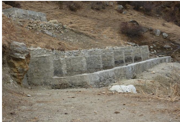
Figure 6-19 An abandoned washing station at Kermi hot springs - local people blame children for cutting the pipes to this station (Author, 2012)
