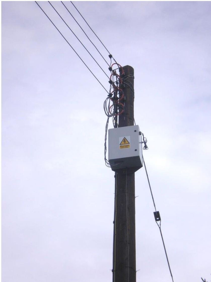
Figure 6.12: Photo of Ametek PQR at pole #15 (Static balancer position)
