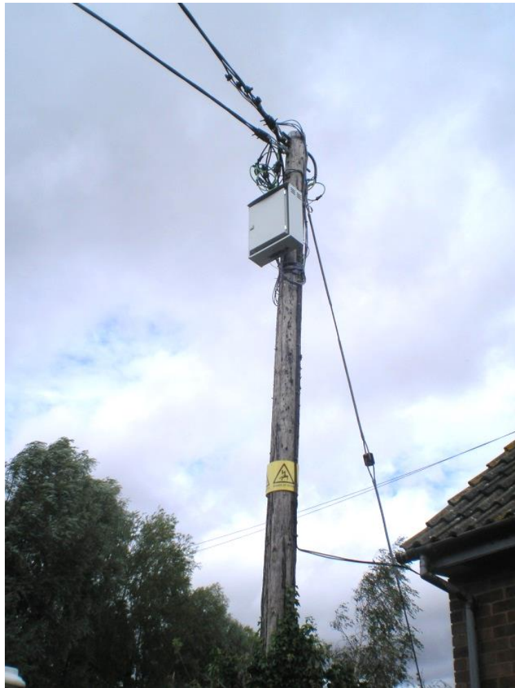
Figure 6.14: Photo of eMS meter at pole #18 (End of feeder)
