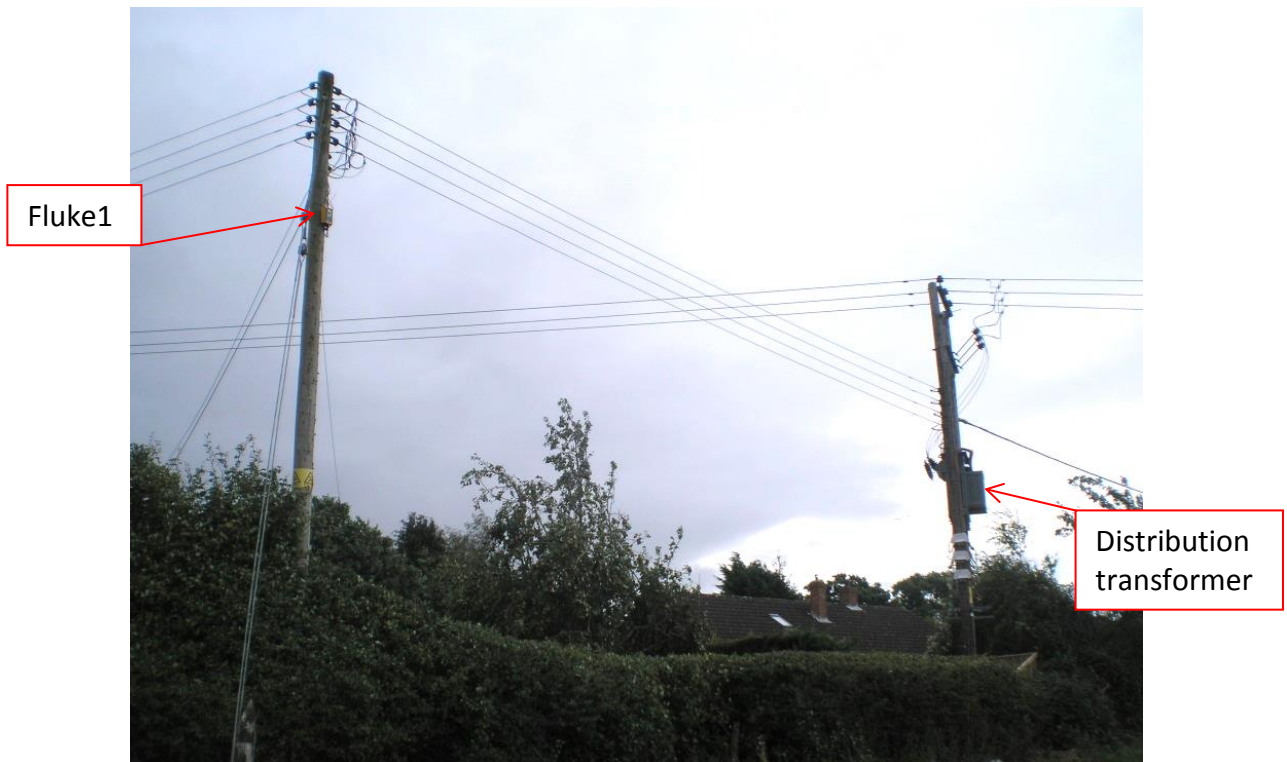
Figure 6.11: Photo showing distribution transformer and Fluke 1 at pole #11 (Start of feeder)
