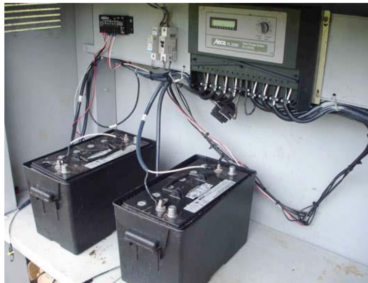
Figure 24. Batteries are charged centrally at the SBCS
