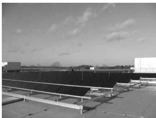
Figure 1: Photograph showing micro-amorphous PV modules on the site in Northern Germany.
