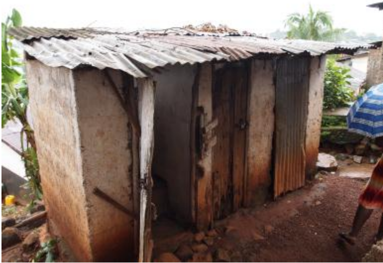
Figure 7: A toilet block with one cubicle for the landlord and two for tenants (Photo credit G Mikhael, Freetown, Sierra Leone)
