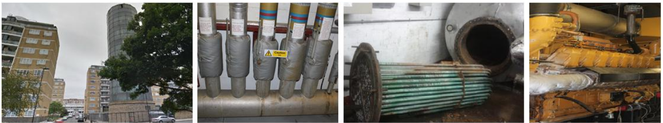
Figure 1: Element of the district heating scheme. Tower block with residences served by the visible accumulator (1), header with flow to the 5 zones in Churchill Gardens (2), a calorifier with “U” bend tubular heat exchangers (3) and a 1.6 MWe CHP engine (4)
