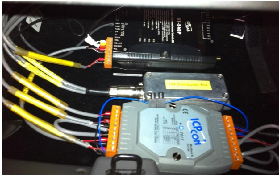
Figure 3.4: Data logger, input module and 12V supply distribution box installed in glovebox
