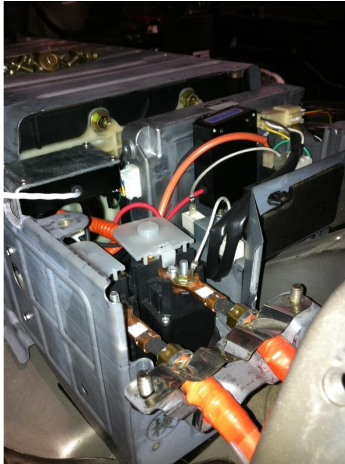
Figure 3.3: HV battery electronics with Isaac current and voltage sensors installed
