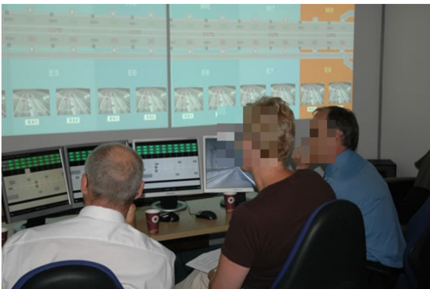
Figure 5. The tunnel control environment during Stage 1 - monitoring hazardous goods during normal operation. Large panel display of layout schematic and CCTV images, desktop simulation of traffic flow and sensor states
