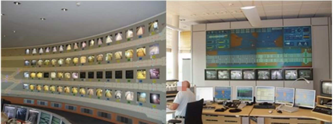
Figure 4. Elbe and Øresund Tunnel control rooms showing tunnel schematic, CCTV images and desktop monitors
