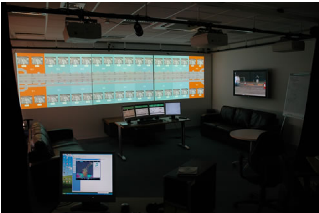
Figure 3. The usability laboratory showing large panel and desktop displays, desktop terminals and simulation control PC (foreground)
