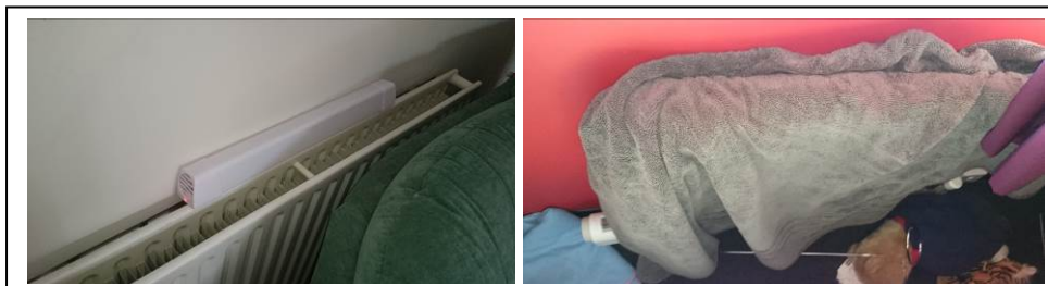
Figure 8a and 8b: Examples of contextual influences on radiators – (left) House 3's lounge radiator with a sofa in close proximity and a battery powered radiator booster; (right) Radiator covered by large bath towel at a study home
