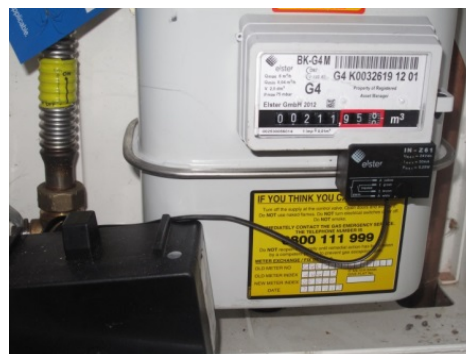
Figure 1. Gas monitoring equipment installed by SMS solutions
