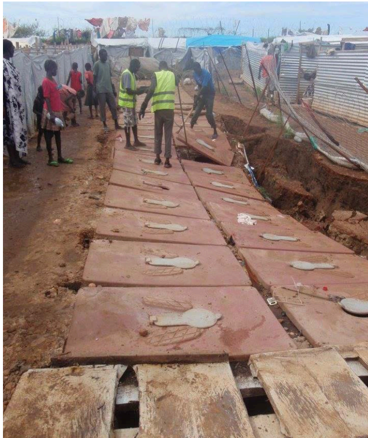
Figure 4 Latrine collapsing before completion
