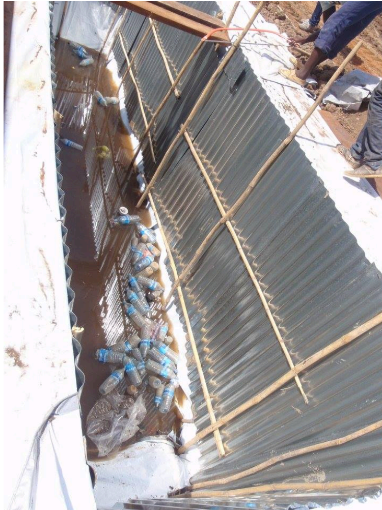
Figure 13 Impermeable liners result in rapid filling of trenches
