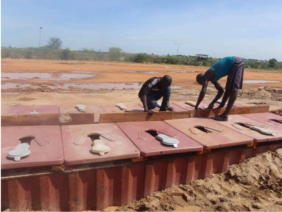
Figure 12 Shipping container being used as a latrine pit
