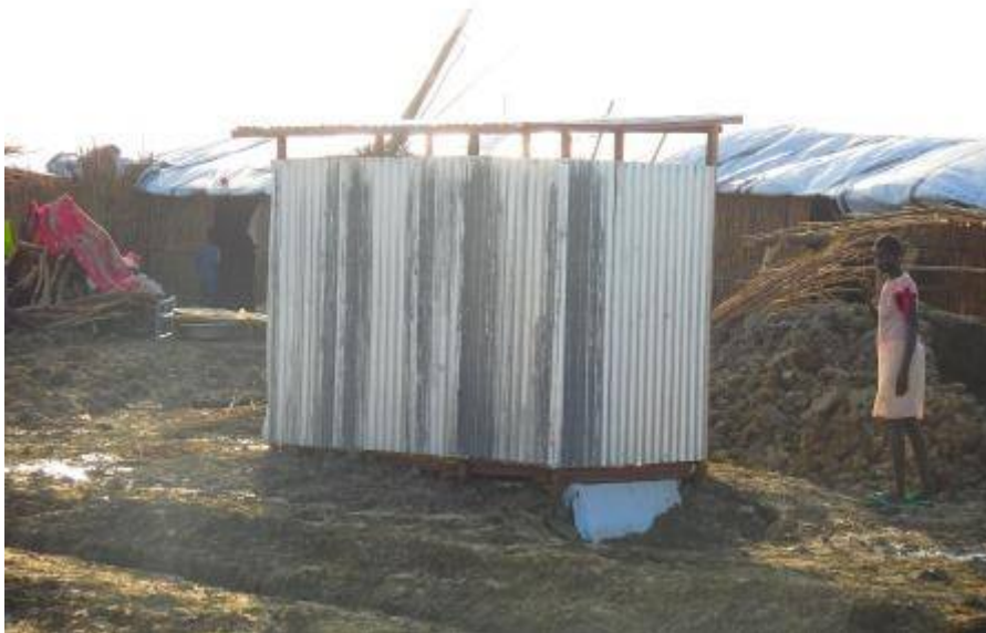
Figure 5 Theft of sandbags from communal latrine surrounds resulting in erosion
