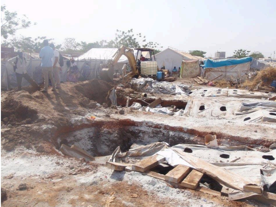
Figure 11 Collapsed latrine trenches
