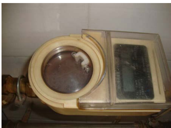
Figure 5 the heat meter installed on input water pipe of heating system in new building
