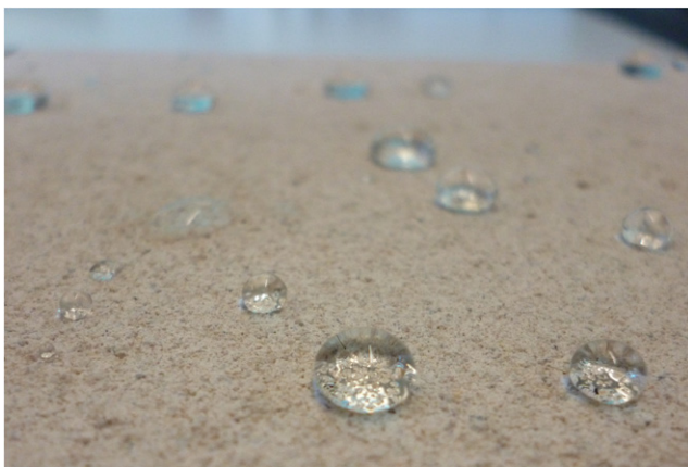
Figure 5. Water drops on a nano-coated concrete brick, showing how the drops form a near-spherical shape
