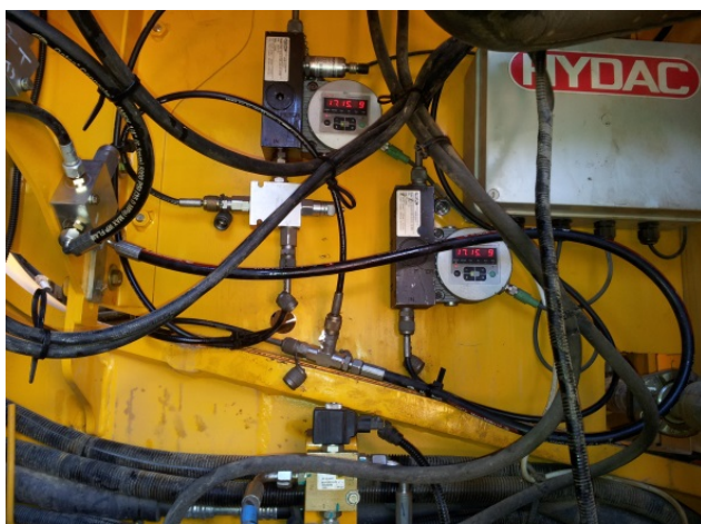
Figure 1 - Particle Sensors and External Data Logger Installations
