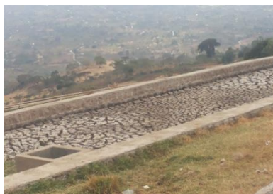
Drying bed at rest
