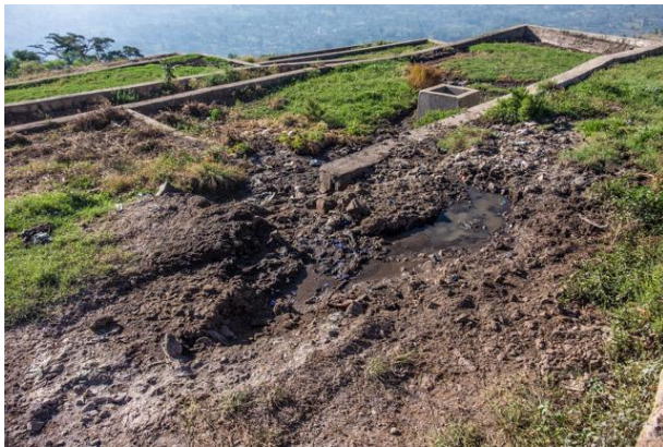
Damaged retaining walls and FS by-passing
