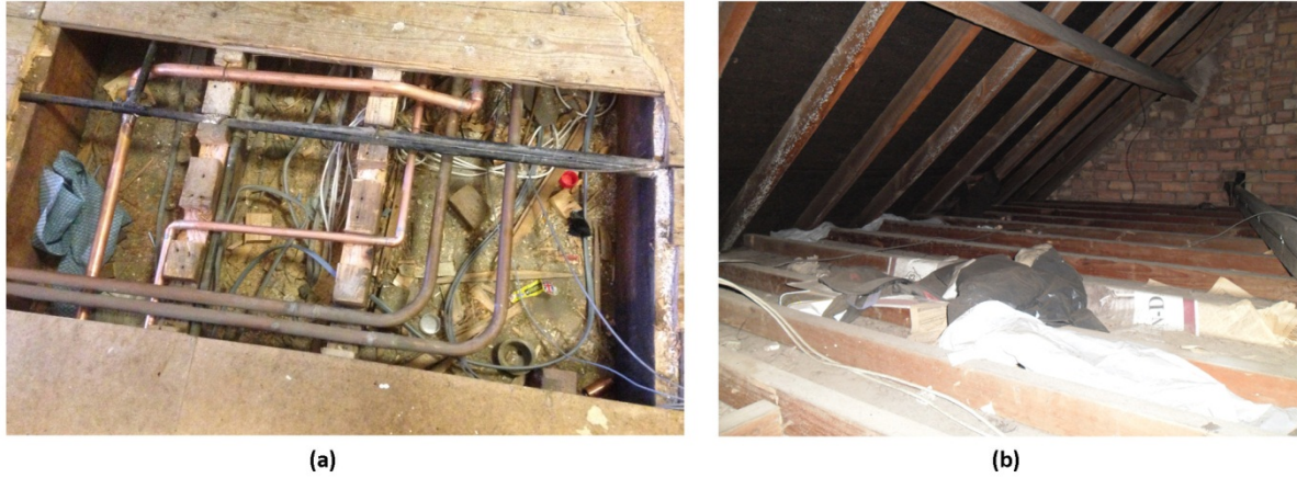
Figure 3-7: Examples of test house inspections for understanding details of construction materials: (a) construction of internal floors; (b) loft (attic) space construction (before removing debris)
