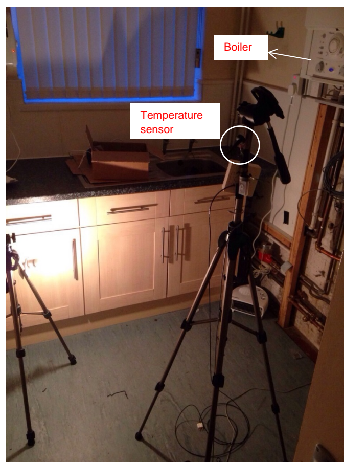
Figure 6-11: Boiler and its uninsulated pipe work and the position of temperature sensor on a tripod in the kitchen of House 2
