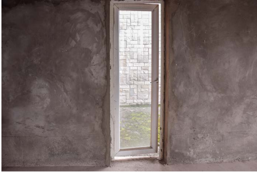
Figure 9 Example of poorly sealed opening
