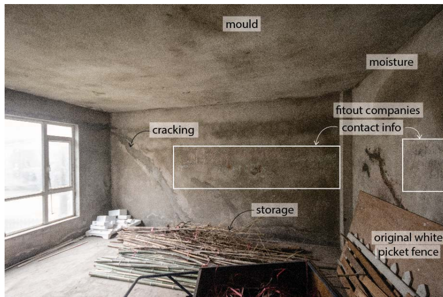
Figure 20 Ground floor with mould, cracking, storage and fit-out company's contact information
