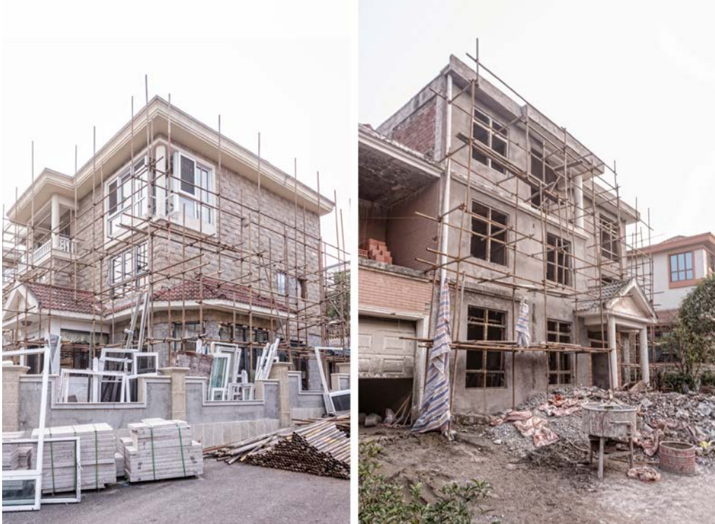
Figure 6 (Re)construction: replacement of windows and lower panels (left) 6 ; stripped back to the concrete structure (right).
