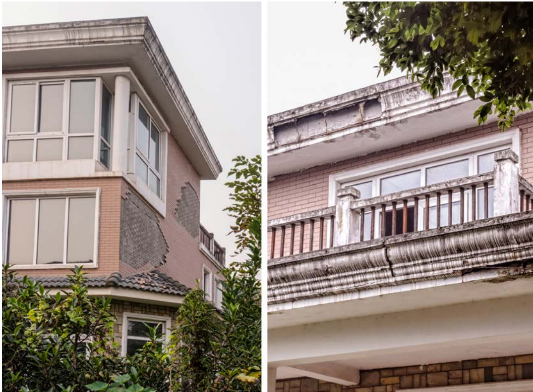
Figure 10 Brick veneer falling off, stained cornice moulding and poorly sealed window openings (left); stained, hollow cornice moulding broken with insufficient metal anchorage exposed (right)
