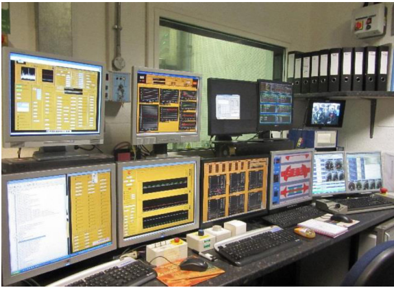
Figure 2. C6.6 engine control room set-up
