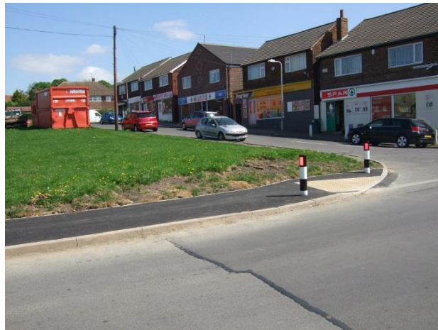
New dropped kerb and path in front of the Spar around green space at Laburnum Parade shops
