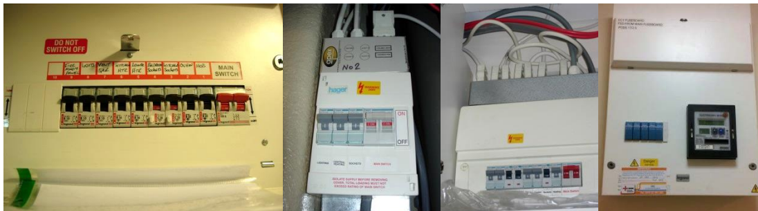
Figure C.1 (far left): Studio flat distribution board
