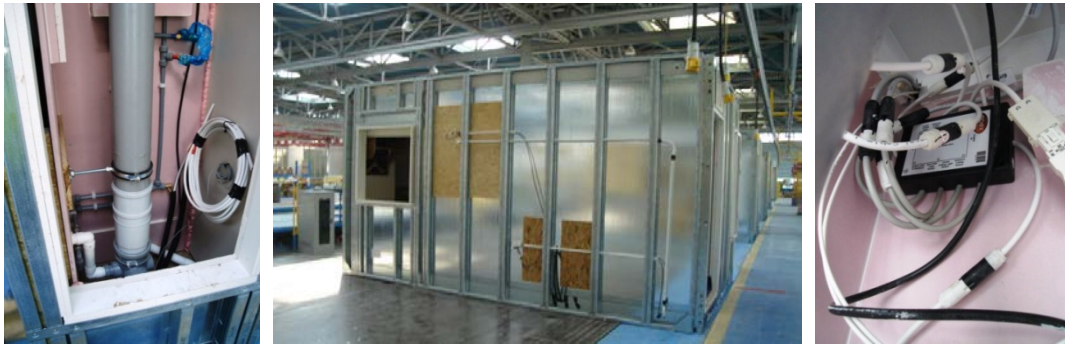
Figure H.18 (left): Bottom of service riser showing shower pod plumbing connected to soil and vent pipe
