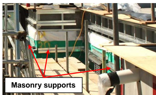
Figure 7.34: Construction site photograph showing numerous steel angles fixed directly to modules [REDACTED] 2012]
