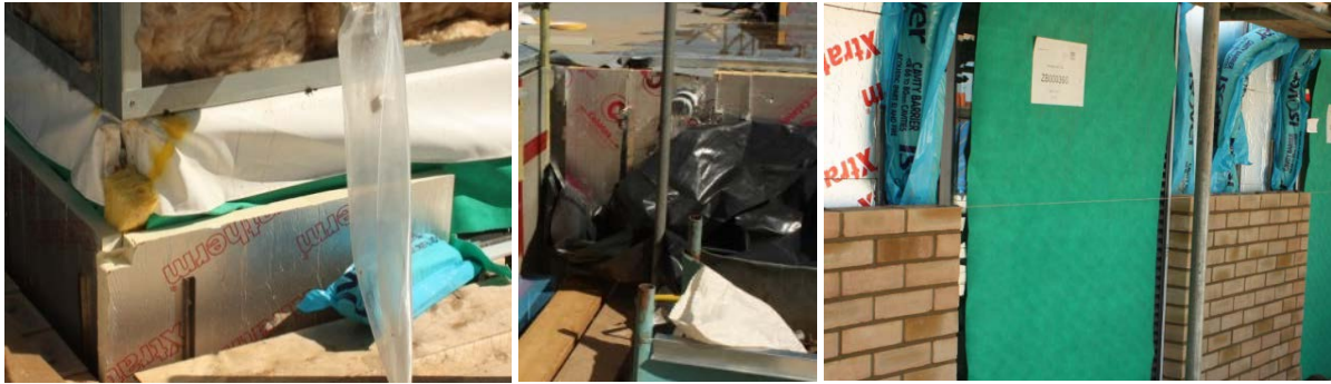
Figure 7.68 (left): Ill-fitting, un-taped rigid insulation and insufficient length of insulation [REDACTED] 2012]
