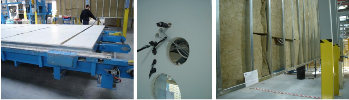
Figure H.5 (left): Ceiling panels with first layer of board fitted, taped and sealed
