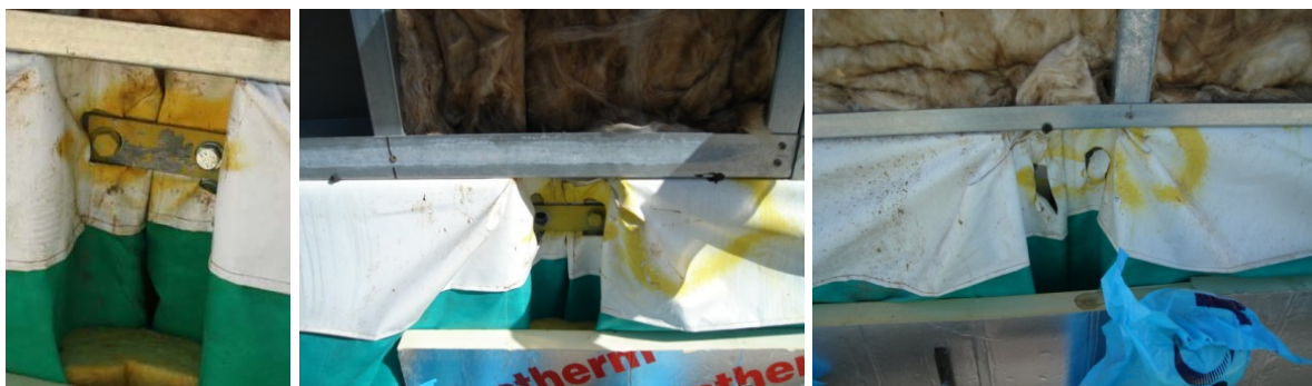
Figure 7.65 (left): Insulation of insufficient length revealing party wall junction behind [REDACTED] 2012]
