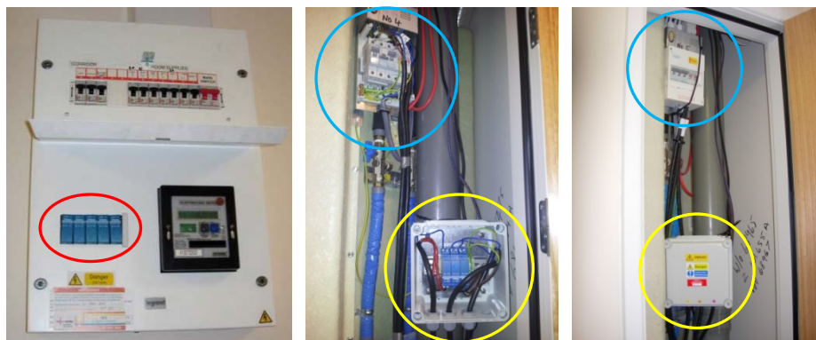
Figure 8.1: Electricity meters installed in Flat 1 DB, the front of the meters are visible (highlighted red)
