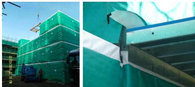
Figure F.3 (left): Module installation on site, showing modules stacked on top of each other [REDACTED] 2012]
