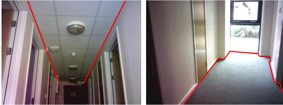
Figure 7.6 (left): Air leakage paths along corridor ceiling indicated in red
