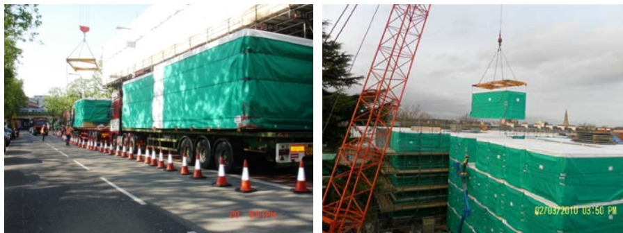
Figure I.4 (left): Site photo: Two lorries on site, the first unloading, the second waiting [REDACTED] 2012]
