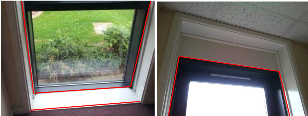
Figure 7.20 (left): Air leakage paths shown in red around bottom of curtain walling
