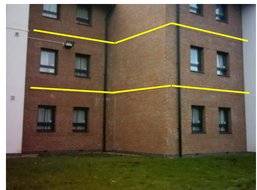
Figure 5.13: Loughborough study – Location of weep holes in brick facade indicated in yellow
