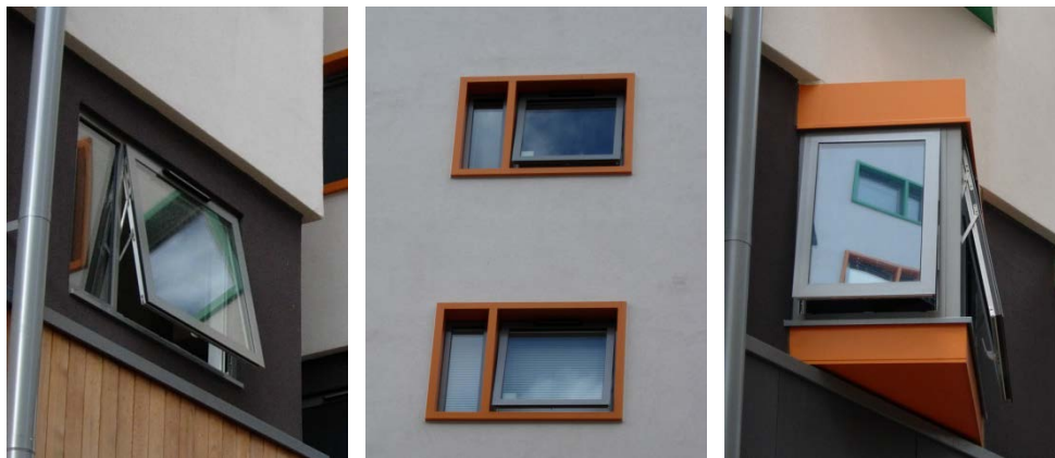
Figure 5.49 (left): London study – Module window not recessed in facade – extent of window opening
