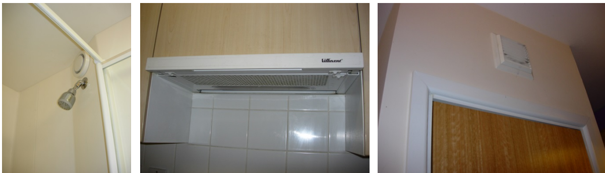
Figure 5.27 (left): Loughborough study – Extract ventilation in showers in bedroom modules
