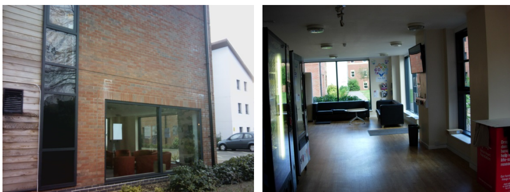
Figure 5.23 (left): Loughborough study: Curtain walling to left and standard window to right
