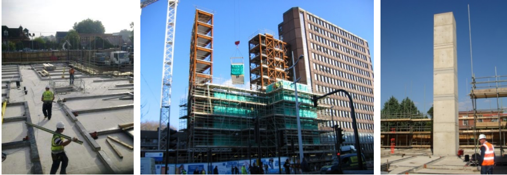
Figure I.1 (left): Site photo: Foundation being prepared on site for module installation [REDACTED] 2012]
