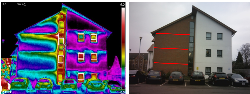
Figure 7.32 (left): IR thermal image shows elevated temperatures due to masonry supports Figure 7.33 (right): Corresponding photograph with masonry support thermal bridges marked in red
