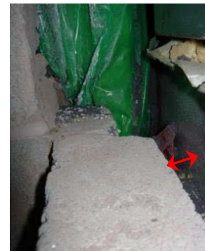
Figure 7.71: Gap between concrete block inner leaf and insulation
