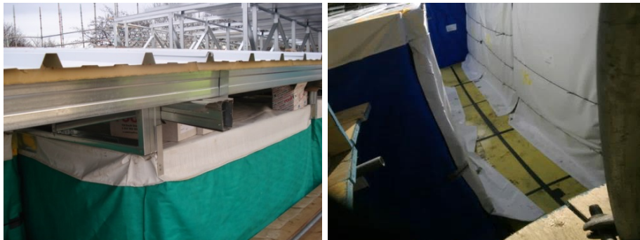
Figure 7.61 (left): Loose fitting breather membrane [REDACTED] 2012]
