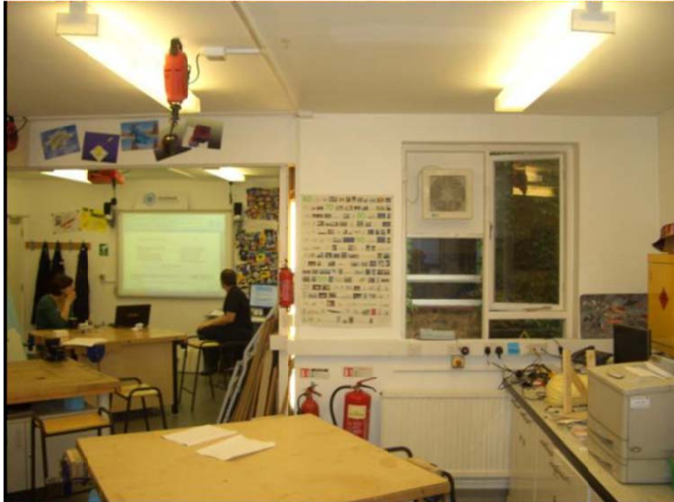
Figure 8-3: View of the classroom showing the supply fan and the adjacent partially open window
