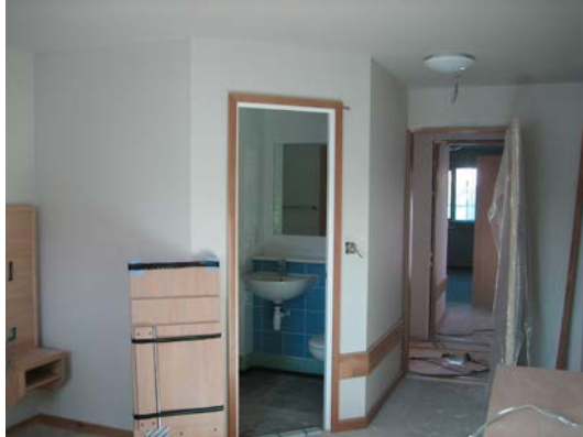
Figure 4.27 Bedroom unit (Gatwick Premier Inn) after installation during secondary fit out (source: author)
