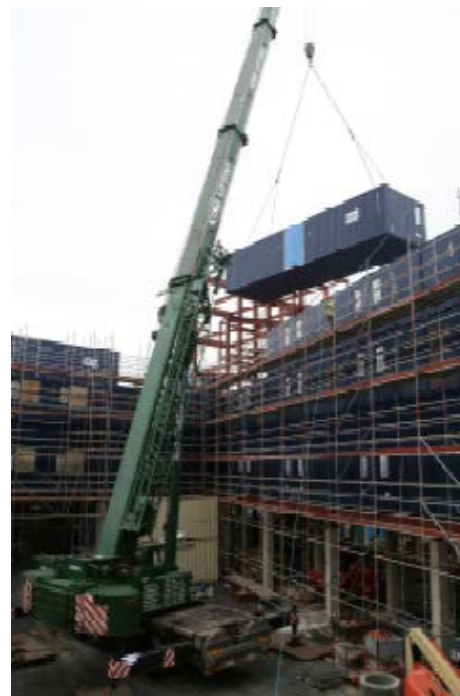
Figure 4.25 Lifting units at Heathrow Travelodge with perimeter scaffold being added (source: author)
