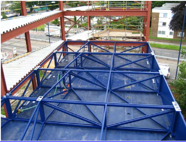
Figure 4.26 Steel make-up pieces to accommodate changes in storey heights between units and main building structure for Heathrow Travelodge (source: author).
