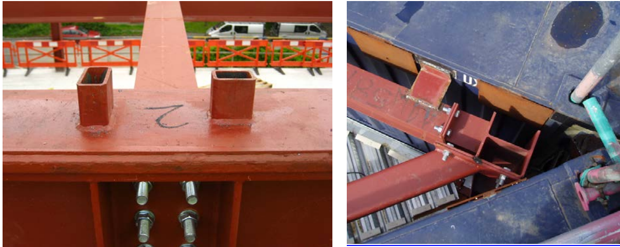
Figure 4.23 Spigots on base steel frame for locating and positioning containers and link plates welded between units and structural frame. (source: Buro Happold).
