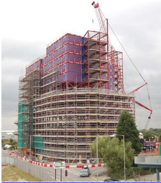
Figure 4.29 Premier Inn, Hull during installation of final level of units (source author)
