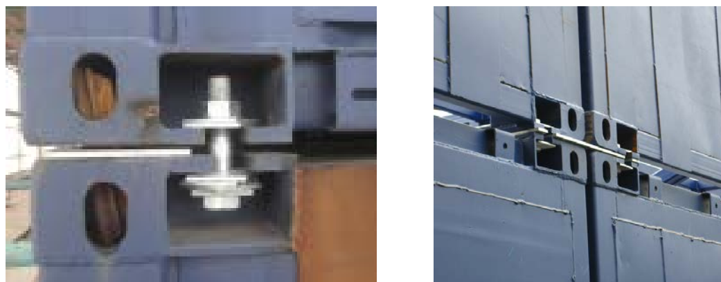
Figure 4.22 Standard vertical bolted connections between units with packing and link plates (source: Buro Happold)
