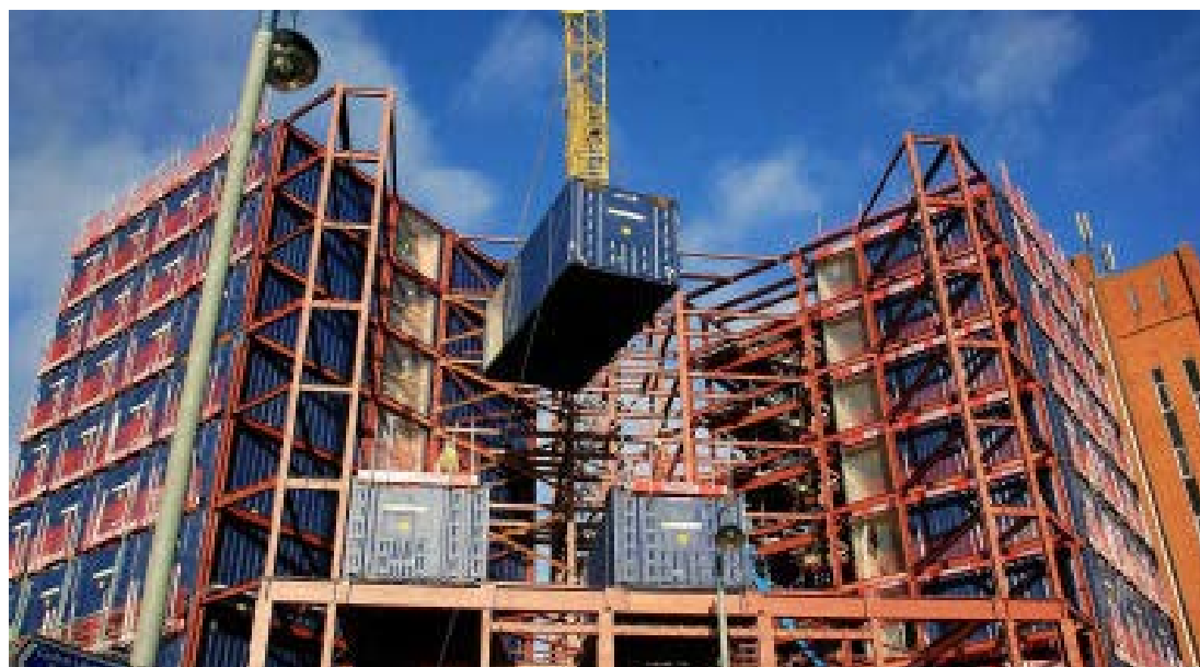
Figure 4.20 ISBU container modules being assembled at the first multi-storey container building for Travelodge, Uxbridge in 2005 (source: author).
