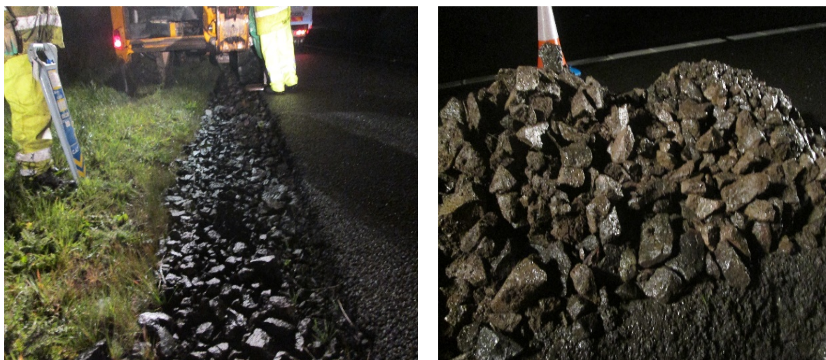
Figure 18 HFD trial M77D on pavement verge M77 and dug out material (exhibiting low levels of fouling)
