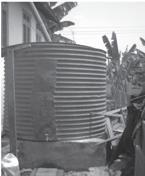
Photograph 1. Rain harvesting system with tap connected to storage tank
