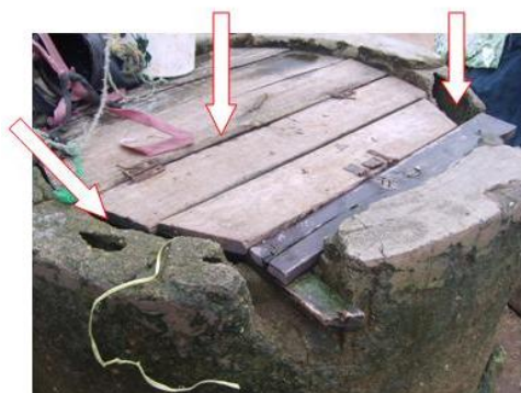
Photograph 1. Fully covered well with gaps within planks, and see-through openings between cover and head wall
