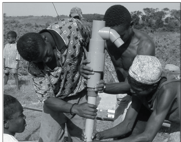
Photograph 2. The pump is installed by the well users themselves
