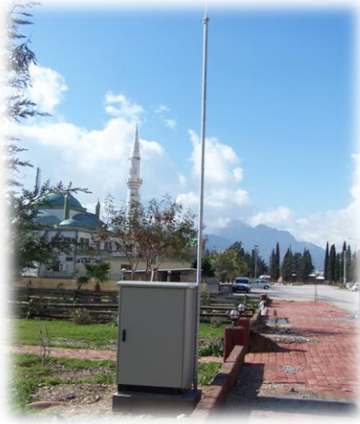
Photograph 1. A typical view of a SCADA station located along a water main in Antalya City
