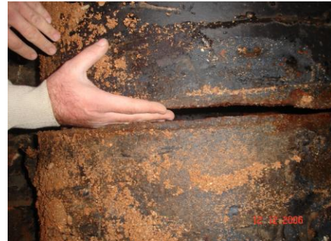
Photograph 4. Crack in the inlet pipe to Caglayan water reservoir in Antalya City detected by carrying out water budget
