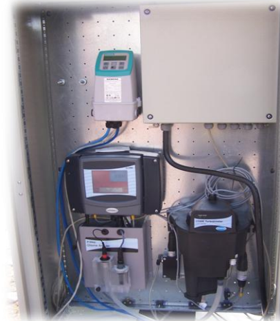
Photograph 2. On-line measurement sensors for temperature, pH, turbidity, electrical conductivity and free residual chlorine
